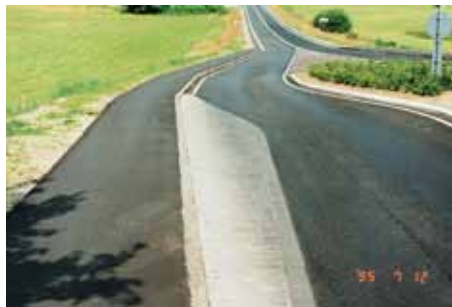
To prevent squeezing, cycle tracks or cycle lanes can be established by a median divider.
