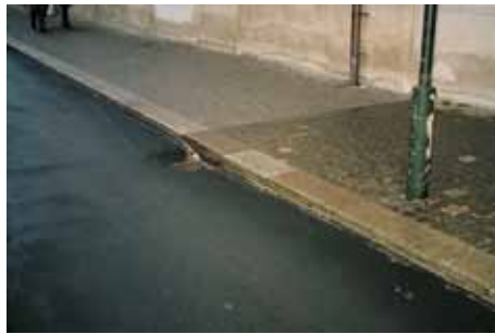
Be careful with drainage construction. The hole here around the grate is much too deep.
